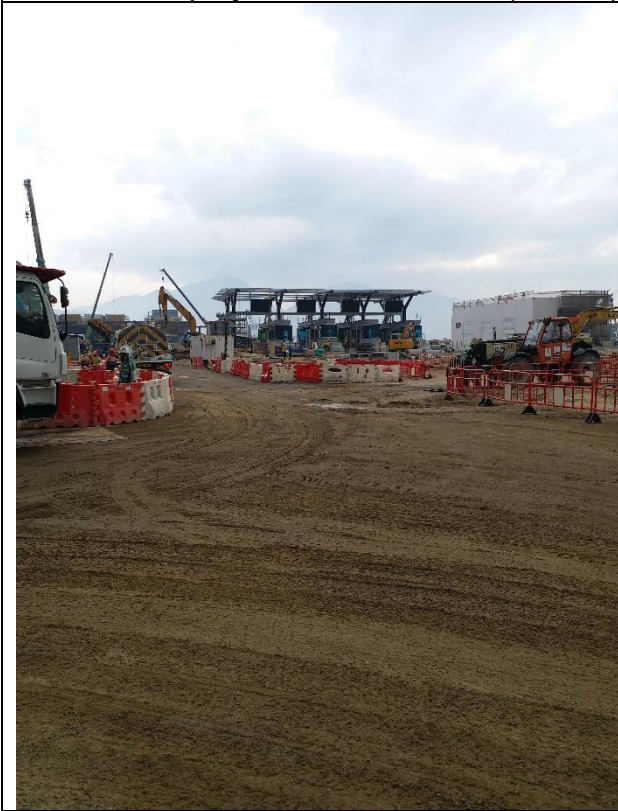
Haul road is wet (Point B)
