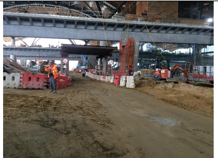
Haul road is wet (Point A)
