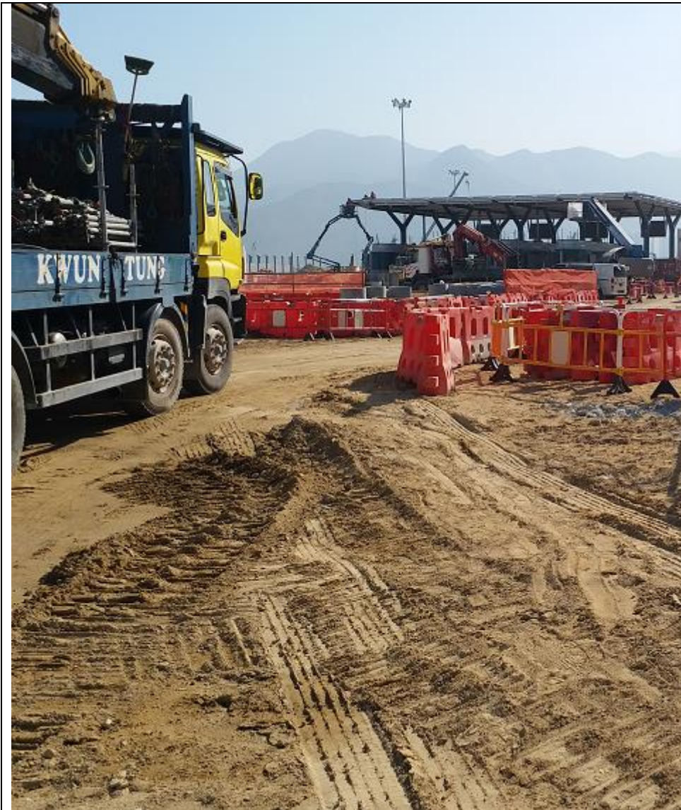
Haul road is wet (Photo taken during site inspection on 27 December 2017)
