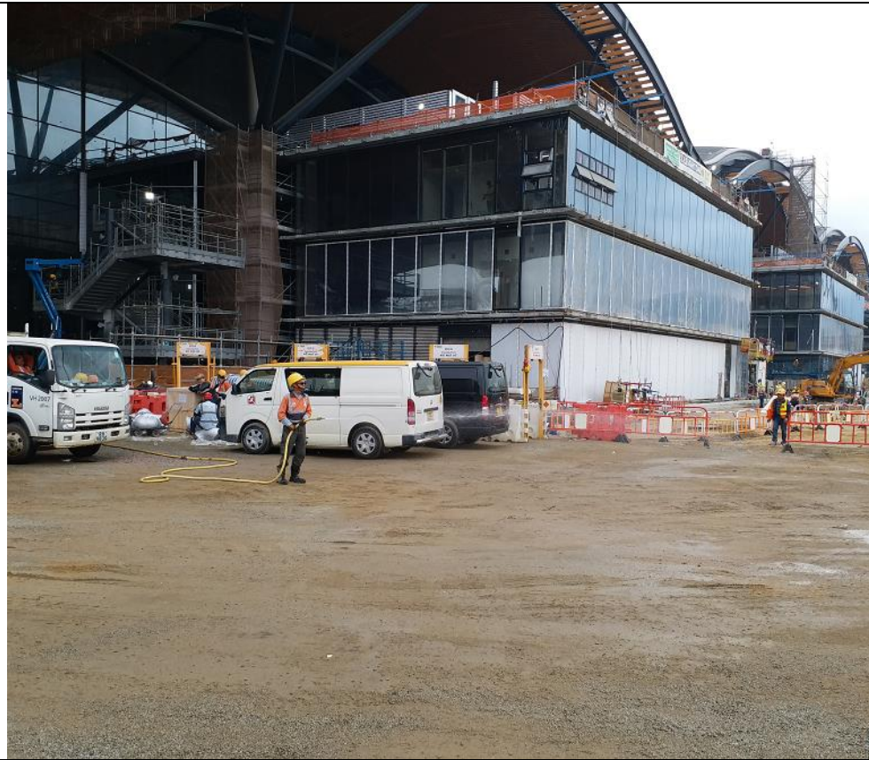
Haul road is wet (Location 1)
