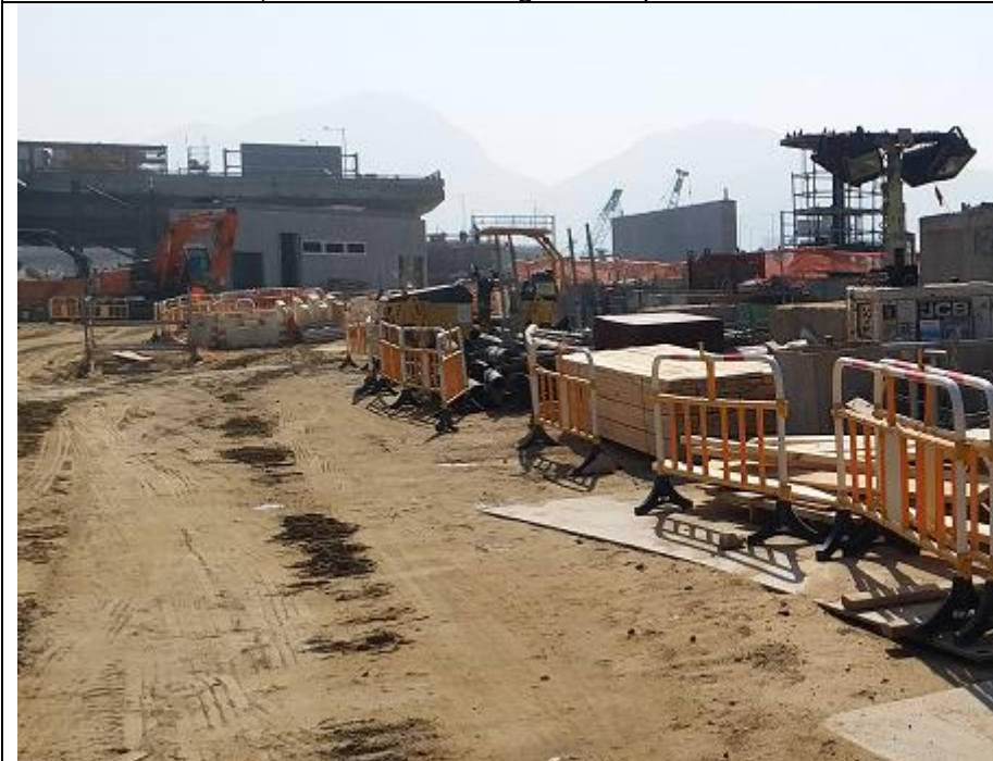
Haul road is wet (Photo taken during site inspection on 27 December 2017)
