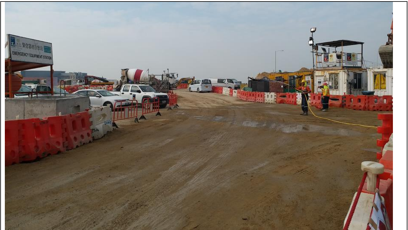
Haul road is wet (Location 1)
