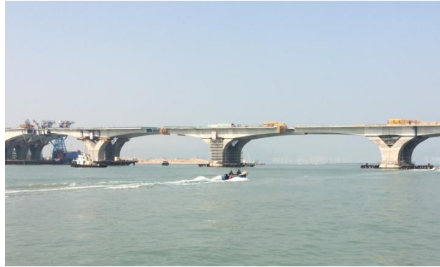
Photo 1 - Mid-Flood at IS8 on 6 December 2017
