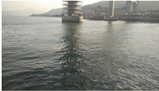
Photo 1 - Mid-Flood at SR4a on 3 January 2018
