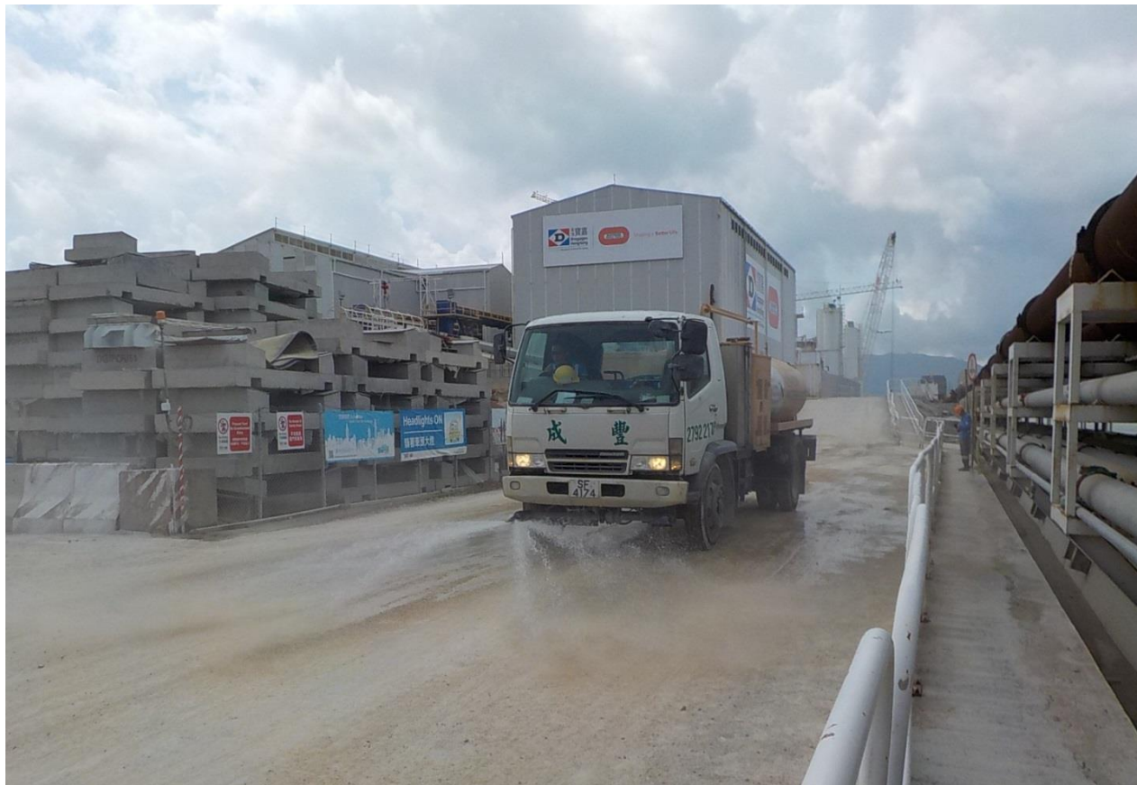
Use of water truck on exposed soil within the Project site and associated work areas. (Works Area Portion N-C)
