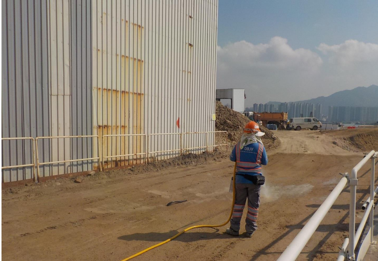
Watering on all exposed soil within the site. (Works Area Portion N-B)
