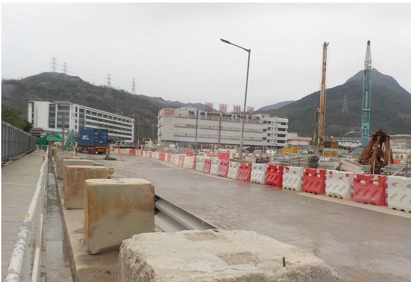
Sprinklers were installed to water the main haul road. (Works Area Portion N-A)
