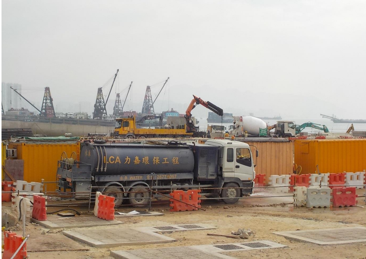
Water truck is used for water spraying to prevent dust. (Works Area Portion N-A)
