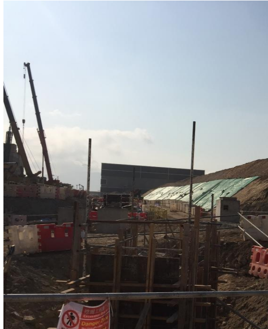
Exposed soil was covered by tarpaulin sheets to prevent dust. (Works Area Portion N-C)
