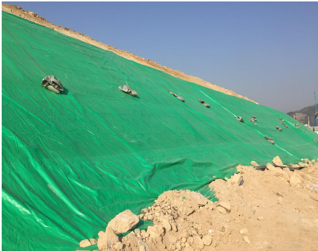
Exposed soil is covered by tarpaulin sheets to prevent dust. (Works Area Portion N-C)
