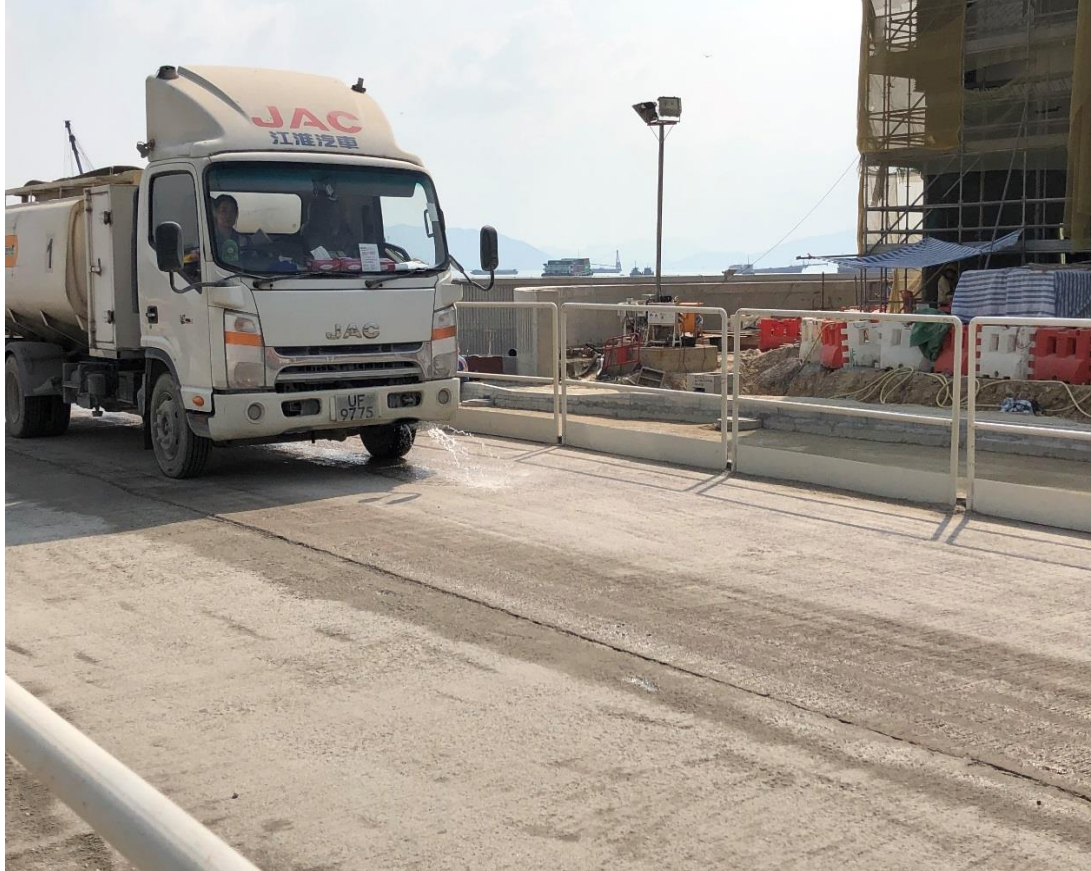
Water truck was used for water spraying to prevent dust. (Works Area Portion N-C)
